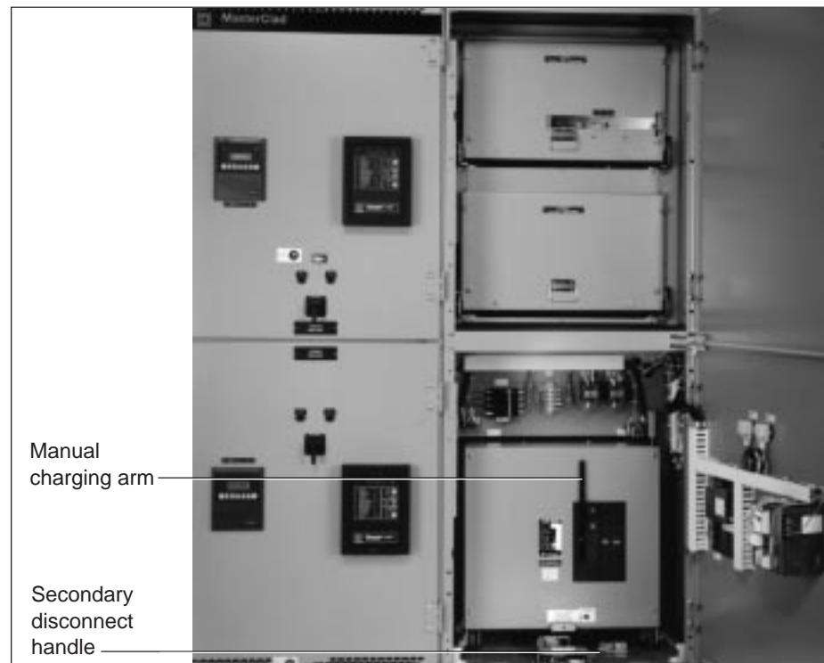
Figure 14: Type VR circuit breaker in test position
