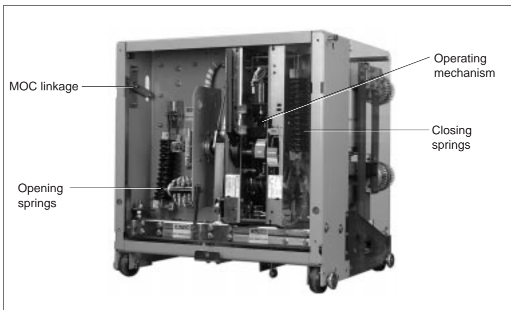
Figure 5: Circuit breaker, right front view without cover
