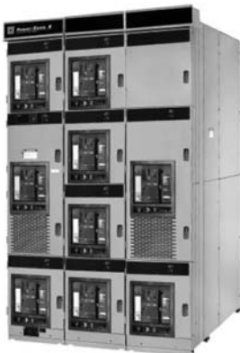
Figure 9-5: Low voltage Switchgear
