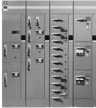
Figure 9-4: Low voltage motor control center
